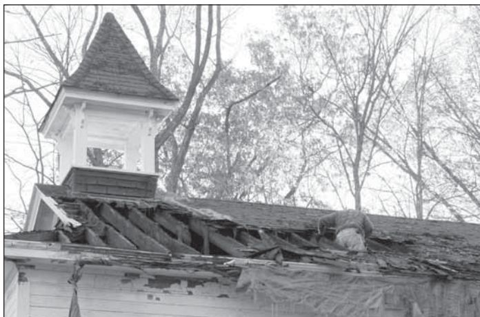
STRUCTURAL SUPPORT and roof deck repairs have been made; but, there is still more to do on the project.
